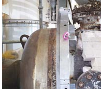
Figure 3 - Vessel presented mounting and clearance issues
